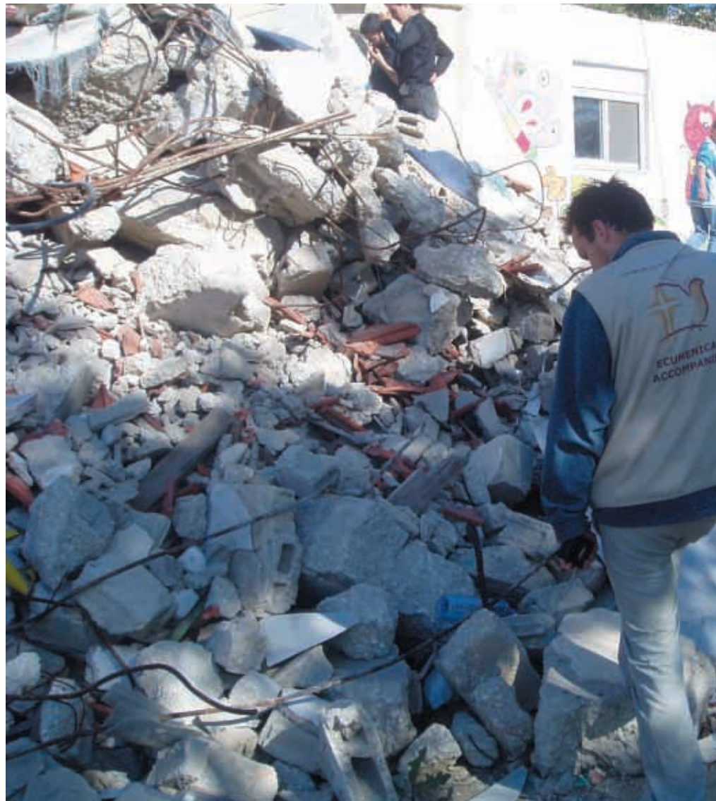
Demolition of a centre for autistic and handicapped children in Jerusalem April 2007, by C. Holtan
