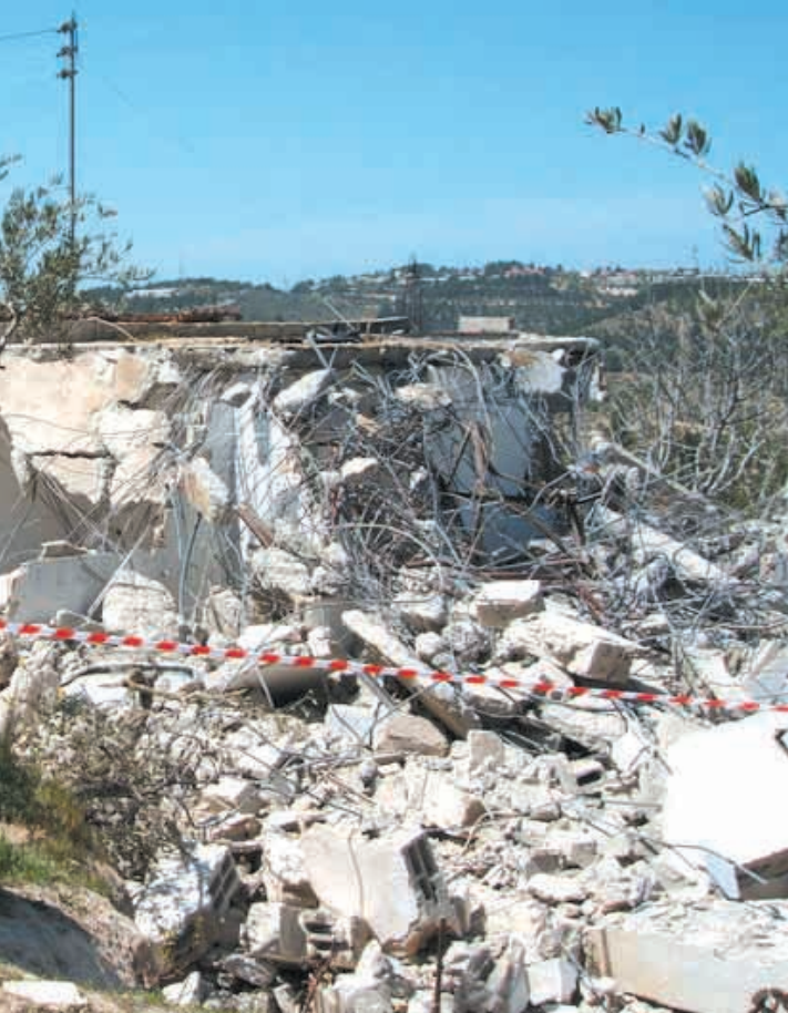
EA in front of a demolished house in Al Walaja, by E.Torjussen
